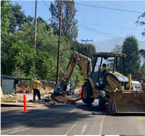
Jack Harms excavates an area of the road where a leak has been located with the assistance of Justin La Point.
