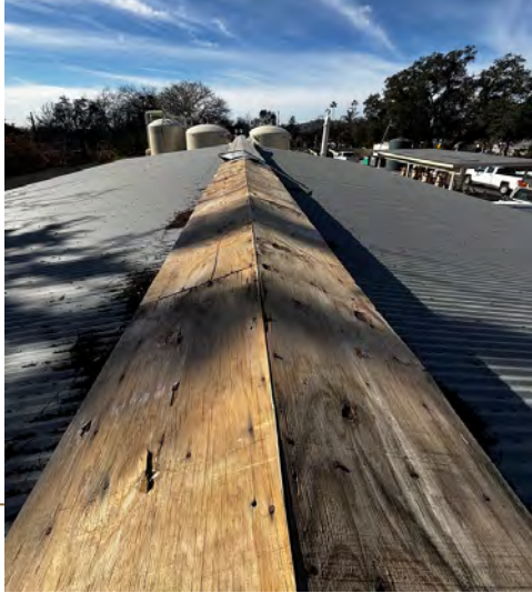
Steel flashing has come loose from the reservoir roof, revealing the wooden frame underneath.
