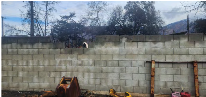
A 125-foot cinder block wall sustained damage due to the intense heat.
