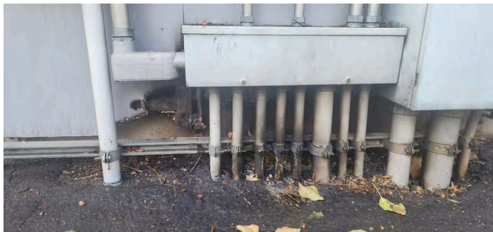
The electrical conduit had been scorched.
